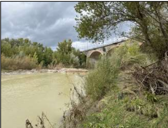
The site of the bombing at Alleron Bridge
